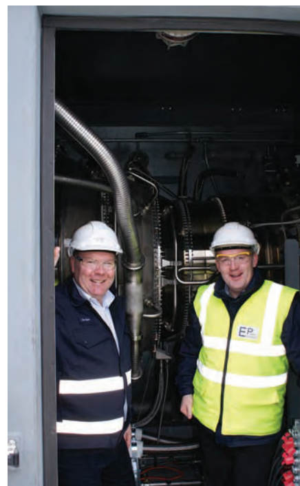
Tom Egan and John Reilly at the new peaking plant at Edenderry.
